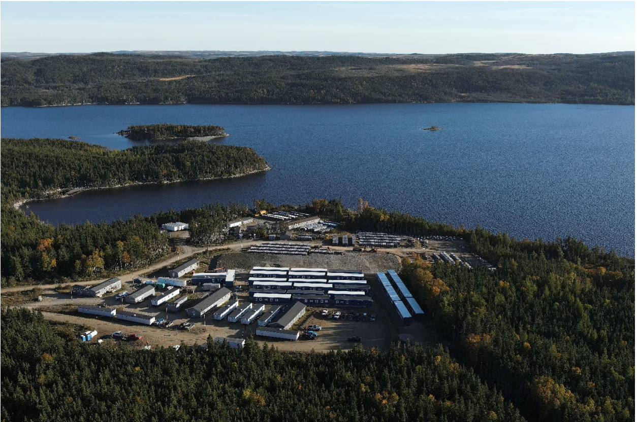
Photo: 120 bed temporary camp installed (top). On-site laydown yard and fuel station (bottom)
