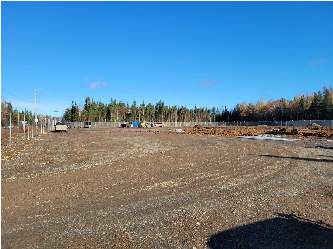
Photo: Construction of the Millertown off-site yard November 2021 (top). In use October 2022 (bottom)
