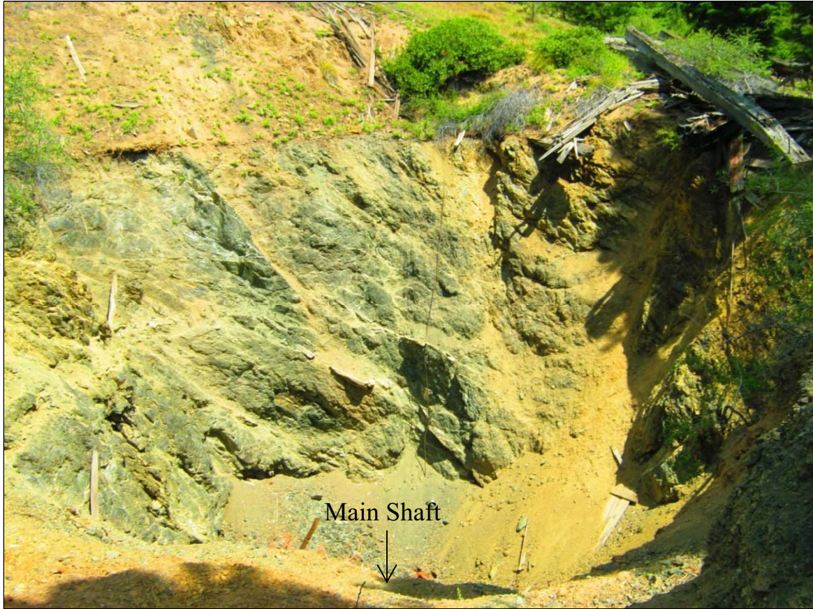
Figure 6.3 Caved-in Main Shaft, Bonanza Mine Property
